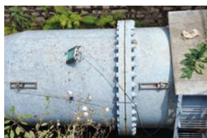
Raw water intake monitoring
